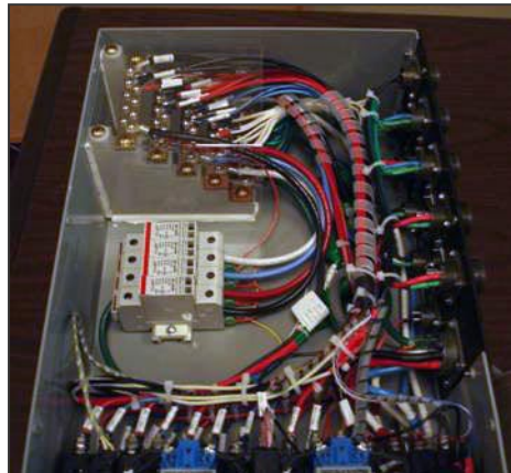
Power Distribution Unit Interior View
